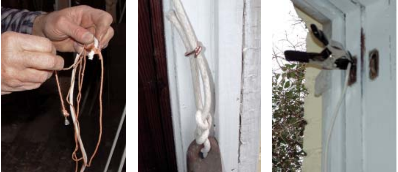
Figure 5. A weighted string helps the author fish new sash cord over the pulley and down to the bottom of the weight box (left). He secures the cord to the sash weight with two half-hitches, then captures the excess cord with a hog ring to prevent it from ever getting snagged in the cavity (center). To allow plenty of slack for attaching cord to sash, he pulls the weight to the top of the cavity and clamps the cord (right).
