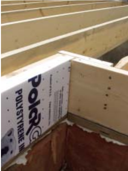
Figure 3. Because the 2x8 mudsill projects 2 inches over the top of the fiberglass insulation board, the author held the rim joist back the same distance on walls where the joists are parallel. This ensures that wall and roof loads from above get transferred directly into the concrete foundation. In addition to a foam sill gasket, he used spray foam to seal the sill to the concrete.
