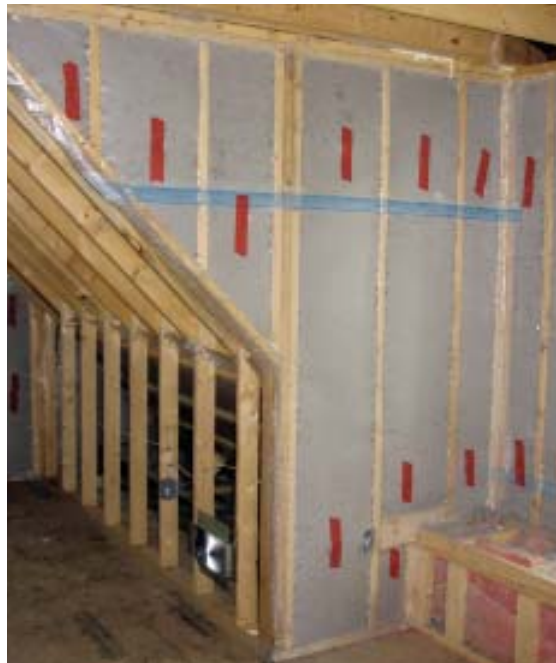
Figure 5. Par/PAC insulation — a high-density blown-in cellulose — provides good air sealing. After stapling up a reinforced poly barrier, the insulation contractor fills each bay through small holes in the plastic sheet, which are subsequently taped up.
