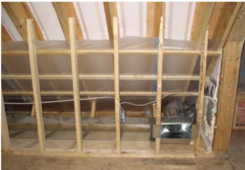
Figure 6. Insulating the roof plane behind knee walls provided conditioned space for running ductwork, which therefore doesn't need to be insulated.
