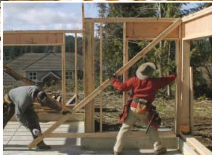
Figure 6. While working on a slab, a carpenter runs the brace in from an angle to avoid marring the concrete floor (left). Below, carpenters rack a wall square by nailing a diagonal to an outrigger fastened to the bottom plates.
