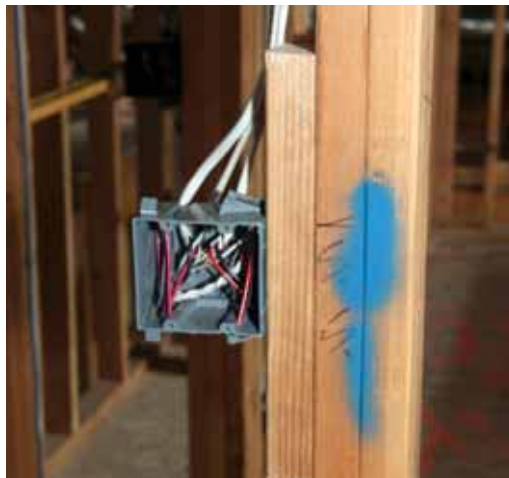
Figure 3. This electrical box was originally installed tight to the king stud, but later was blocked to provide clearance between the cover plate and casing.
