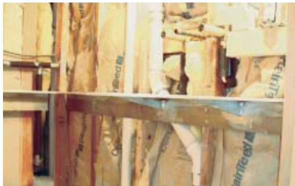
Figure 3. Unlike the rest of the bracket, the gussets beneath the sink are not completely hidden. The aluminum fabricator felt the additional strength was necessary to prevent flexing, which could crack the countertop at its weakest point.
