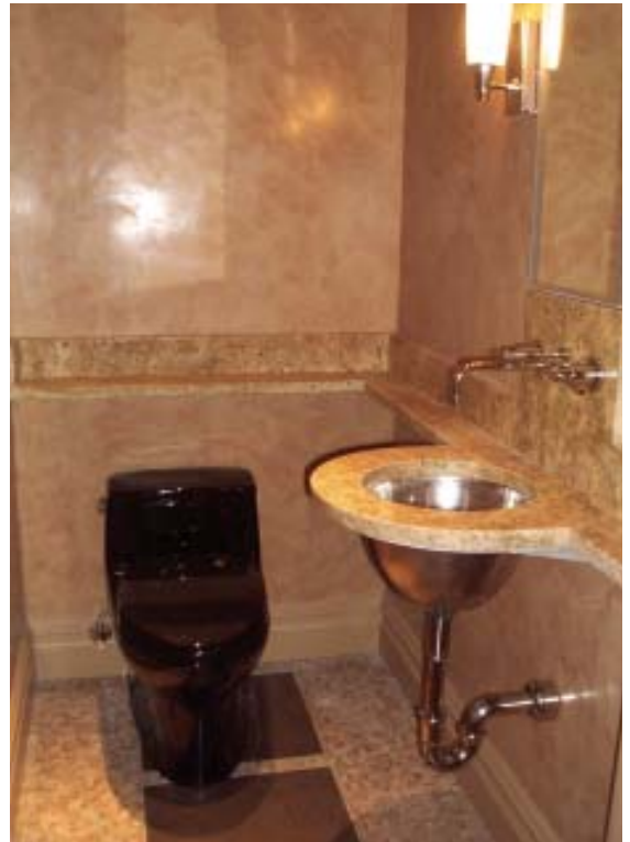
Figure 1. A custom-fabricated aluminum bracket — rather than a vanity — supports this stone countertop, maximizing the tiny powder room's floor space.
