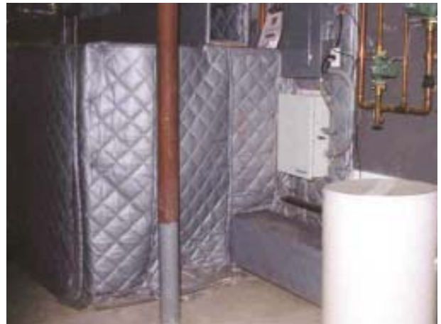
Figure 10. With basements increasingly used for living space, heating and air-conditioning noise is a growing problem. Adding acoustic controls is a good idea, but the products installed in mechanical rooms must be Class-A fire-rated.
