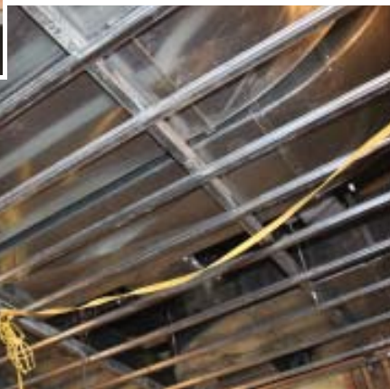
Figure 3. Controlling structure-borne noise requires acoustic isolation or decoupling of the finished space from the framing and other rigid materials. This can be done by using double-stud framing to build a “room within a room” or with specialty products such as these spring isolators (top). On the ceiling of this room, spring isolators support heavy-gauge steel framing (above) that will ultimately be covered with a layer of \frac{3}{4} -inch plywood, a layer of mass-loaded vinyl, and then drywall. Multiple pipes and ducts didn't leave a lot of room for regularly spaced mounting hardware in this high-end home theater, so spring isolators — which generally have a higher load capacity than other types of isolation hardware — were a good choice.
