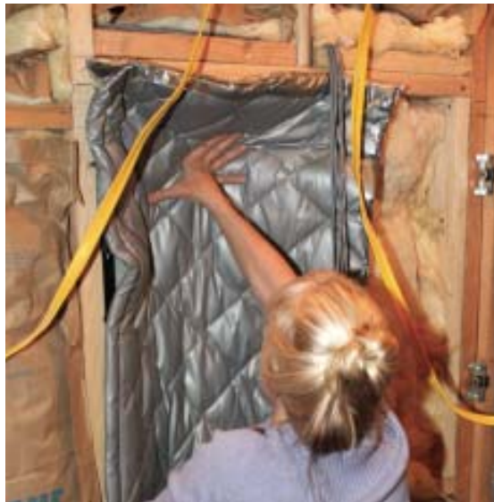
Figure 8. Most dedicated home theaters have built-in speakers. To contain noise and low-frequency vibrations, the author often lines the cavity behind the speakers with a special quilted fiberglass insulation that contains a high-density loaded-vinyl barrier.
