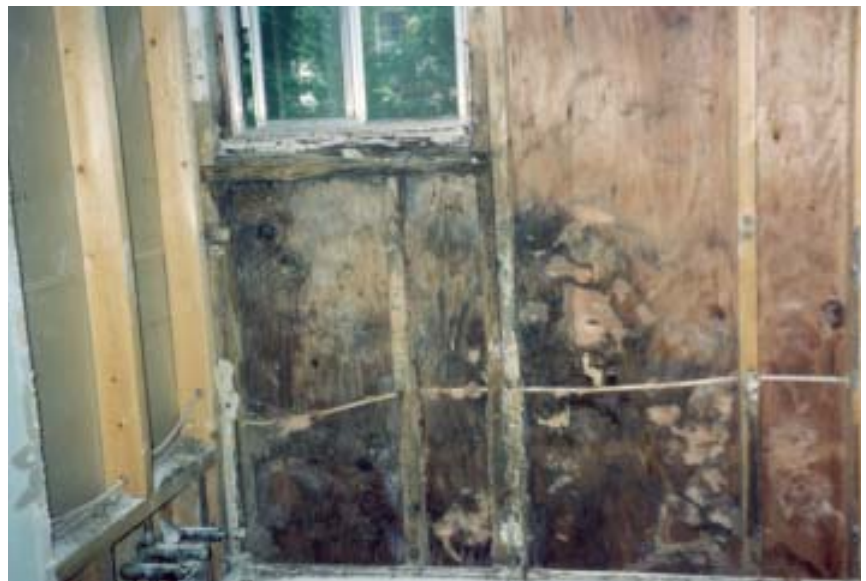
Figure 1. In many bathrooms, the only available location for a window is over the tub. But when the window isn't designed to shed water on both the exterior and interior, moisture can penetrate the walls and cause rot, mold, and other damage.
