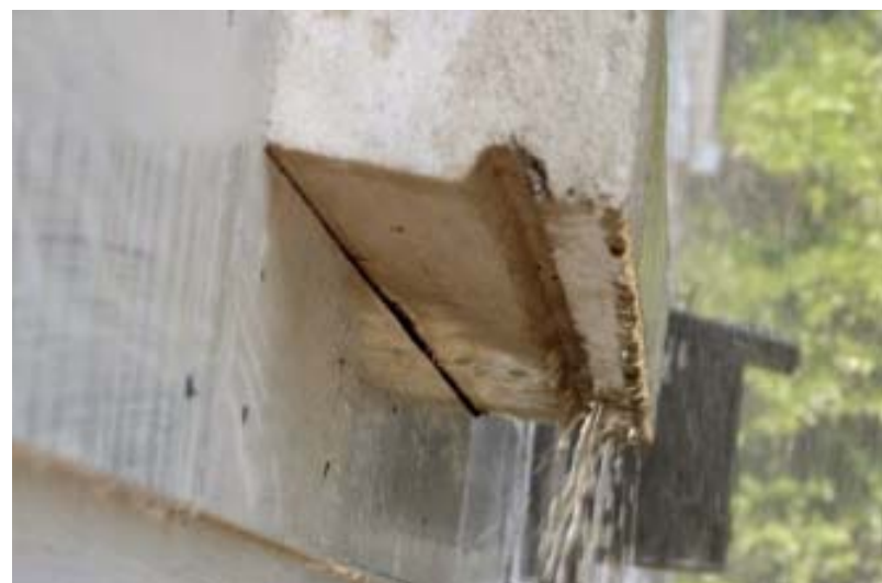
Figure 3. The cast-in-place concrete sill provides a level, stable foundation for the glass-block window (top). It was cast with a drip channel that prevents water from seeping along the underside into the building envelope (above).
