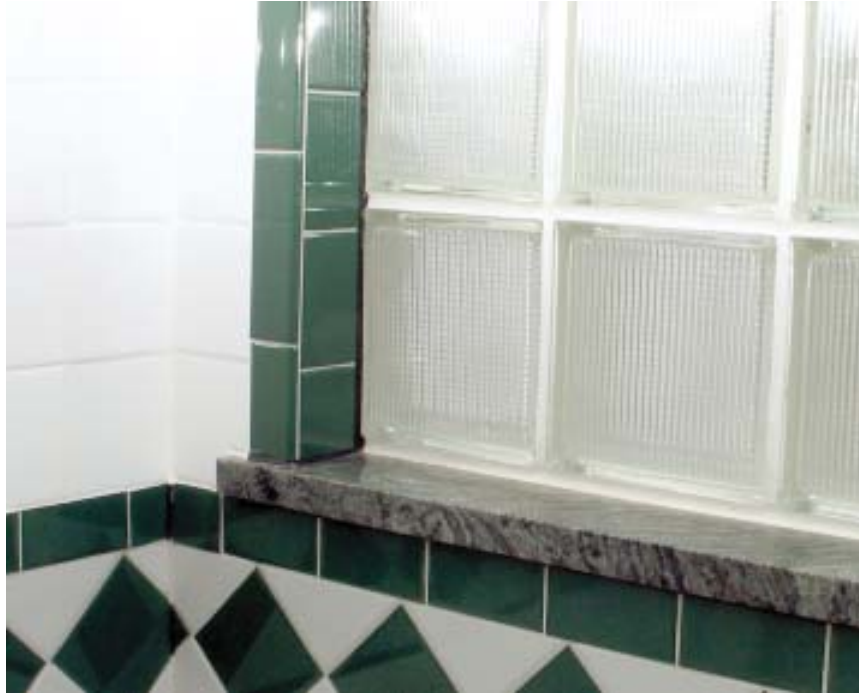
Figure 5. Installed on a bed of Type S masonry cement, the granite slab sill angles down slightly — toward the tub and away from the glass-block panel — for drainage.
