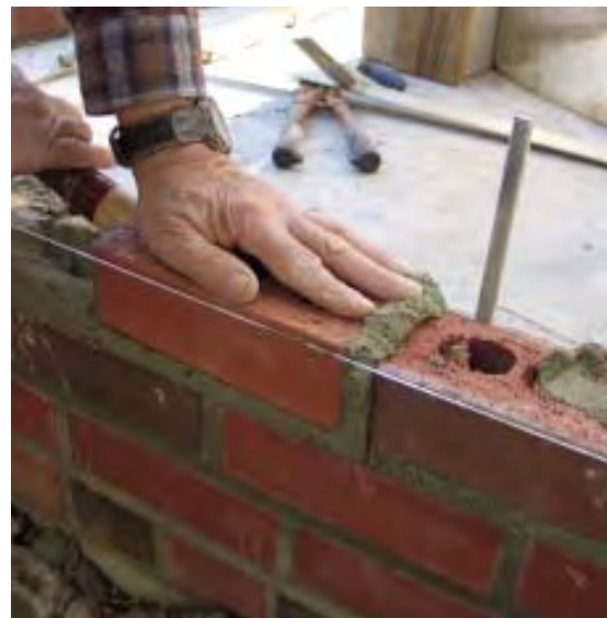
Figure 6. Though partially filled head joints (top) are all too commonly seen in the field, head joints should be completely packed with mortar to prevent water intrusion (above). The author butters the end of each brick before setting it, then taps the brick with his trowel to compress the mortar and align the brick with his layout marks, which are marked on the course below.
