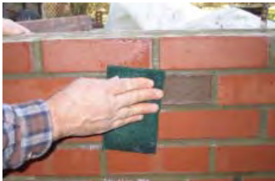
Figure 8. Synthetic steel wool works well for cleaning smooth-faced brick. The author scrubs carefully with a dry pad while the joints are still soft, then gives a more aggressive cleaning the following day with water.
