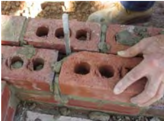
Figure 7. To hold down the treated mudsill, the author installs L-shaped anchor bolts, cutting the bricks to fit around the bolts and filling any voids with mortar.
