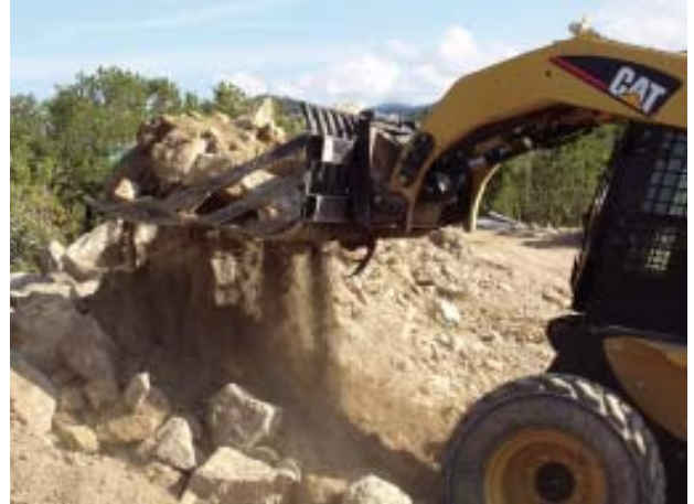
Figure 7. The author frequently uses a rock rake ($1,000) to prepare soil for backfilling utility trenches and final grading. The tool sifts out large- and medium-sized rocks so they won't damage underground utilities; the separated rocks can often be used for other purposes. The rake can also eliminate the need to import clean fill for backfill.
