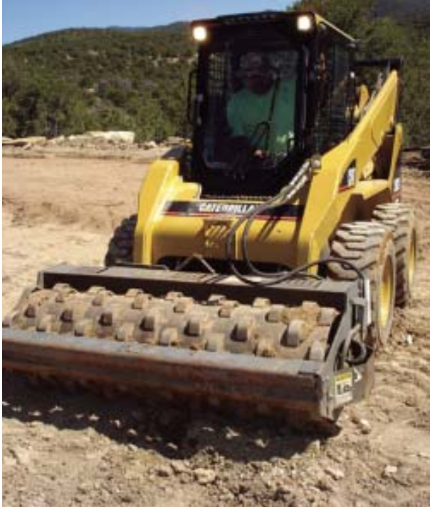
Figure 6. Compacting soil while backfilling or building roads on residential sites is seldom given the attention it deserves. A vibratory roller ($10,000) makes the process faster and relatively foolproof.
