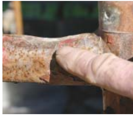
Figure 15. This bent cross-member could compromise the structural integrity of the entire frame, so it was removed from service (far left). The author points to tubing dented by an attempt to force-fit together unlike or damaged frame units (left).
