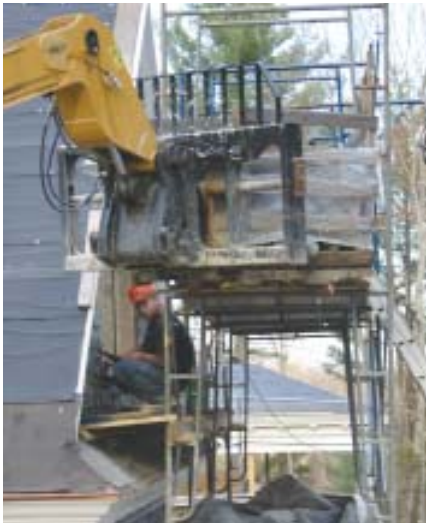
Figure 6. Mobile lifts and other heavy equipment can overload scaffolding in a single drop. Always transfer materials by hand and distribute the load evenly over the platform.
