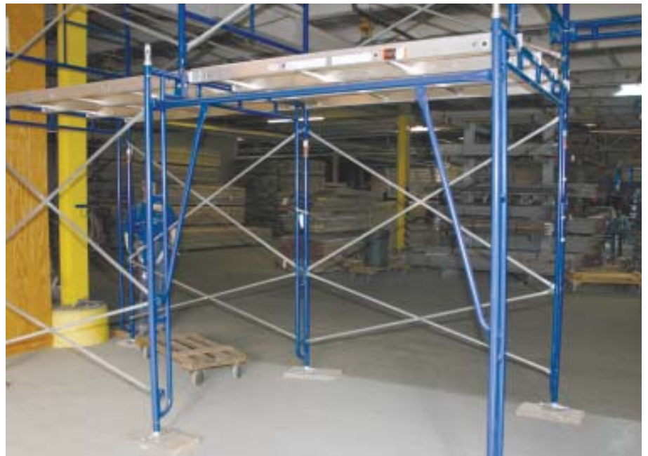
Figure 12. Don't submit to the temptation to remove or simply not install braces on the working side of a scaffold. Instead, use straddle frames, which replace the brace function while still providing good access to the work surface. These walk-through frames allow unimpeded traffic flow beneath the staging.
