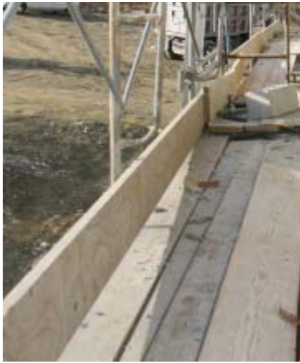
Figure 9. Falling objects present a huge safety hazard on the job site. Toeboards prevent tools and materials from being knocked off the scaffold and should always be installed before loading and using the platform. Full-width planking prevents both drops and falls.
