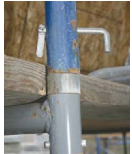
Figure 8. Wind uplift and frame separation are serious concerns. Never omit the toggle pins that secure both ends of the couplers between frames.
