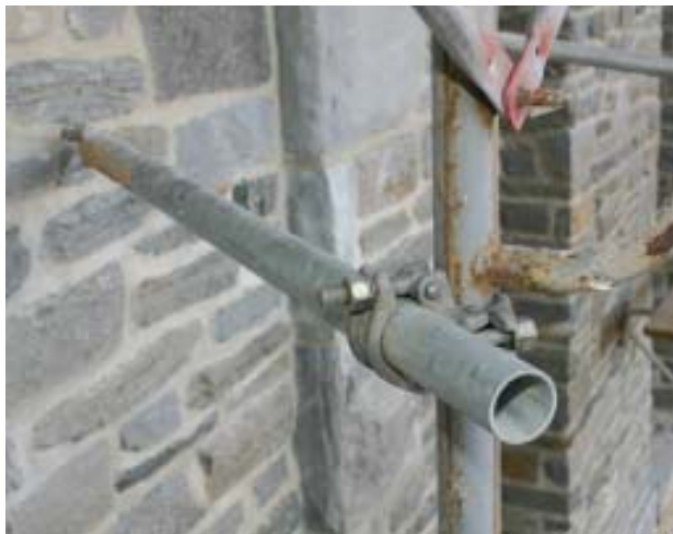
Figure 2. Rigid ties prevent toppling as scaffold height increases. As a general rule, ties must be used when scaffolding reaches a height four times the narrowest dimension of the base frame (20 feet for common 5x7 frames). In masonry, the author uses expanding anchors to make the attachment.
