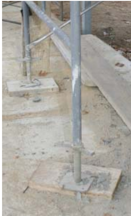
Figure 1. Screw jacks should be considered basic equipment for safe, level setup (right). Although the steel base plates distribute the weight to help prevent tip-overs, they should never be used without a minimum 1-square-foot wood mudsill. Stability is enhanced when frame legs share a common mudsill (far right).
