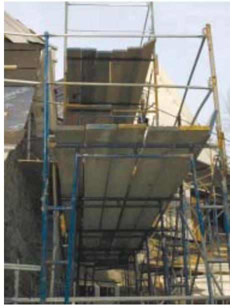
Figure 11. Work platforms higher than 10 feet above the base level must have two parallel guardrails placed approximately 19 and 42 inches above the work platform to prevent falls (far left). Even platform ends must be closed (left). The full platform and high railings on this slate roofing job supply an unbeatable degree of comfort, convenience, and efficiency.
