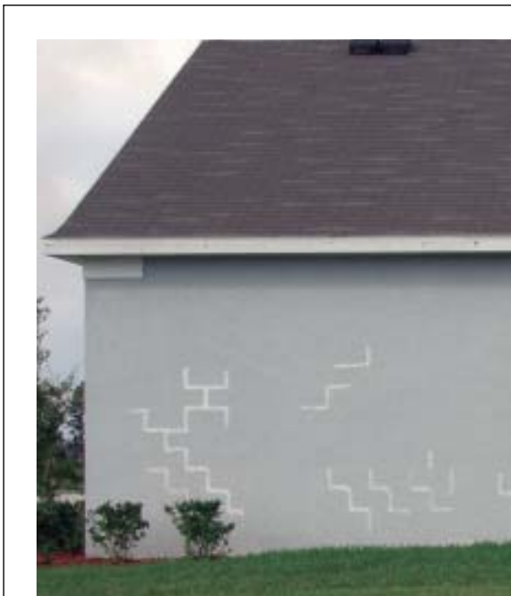
Figure 3. Houses shift after construction as supporting soils consolidate and materials change size with changing temperature and moisture content. This movement of substrates, though typical and expected, inevitably brings about some cracking in brittle surfaces like stucco, creating the need for ongoing maintenance and repair in the early years of a building's service life.
