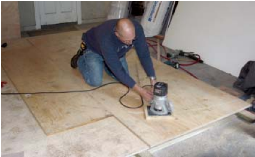
Figure 1. To make a layout table, the author fastened full sheets of \frac{3}{4} -inch plywood to 2x4 sleepers, then used a trammel to draw and cut out the parts of the portico, starting with the roof sheathing shown here.
