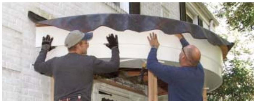
Figure 5. Two layers of PVC trim cover a double layer of 1/4-inch curved plywood subfascia. The upper layer of fascia trim hides the stainless steel screws fastening the lower layer and provides a ground for the PVC dentil molding.
