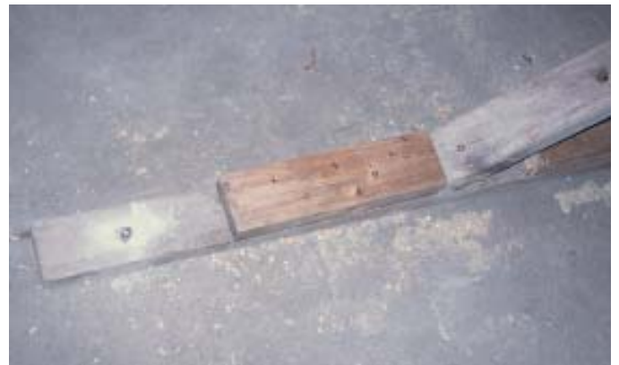
Figure 6. After tightening the nuts on the steel channel, the author placed a grid of 1/2-inch rebar (top left) behind a carefully braced one-sided form (top right). To prevent the form from moving, the kickers along the floor were secured with 6-inch lengths of rebar driven into drilled holes in the existing slab every 18 inches (above).
