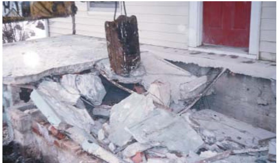
Figure 2. To avoid the risk of running a jackhammer on an elevated slab, the excavation sub used an improvised ram to break up the concrete. When the slab and foundation were gone, the smaller pieces close to the house were removed with a sledgehammer.
