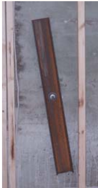
Figure 3. Like a giant plate washer, steel C-channel (right) placed across the existing foundation's weak area spreads the resisting force from the concrete deadman outside. Threaded rod passing through the foundation wall (below left) is welded to steel rods that hook around the rebar in the deadman (below right).
