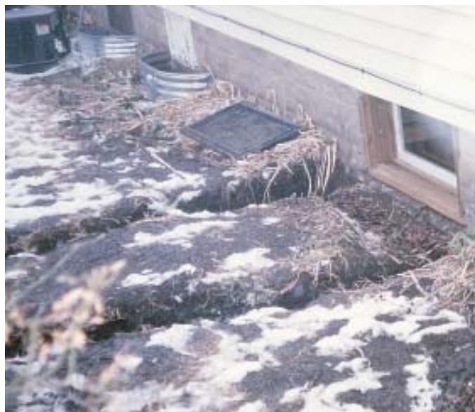
Figure 5. Four-foot-deep trenches (above) partially filled with concrete anchor the steel channel “plate washer” in this section of the foundation. The new reinforced concrete wall, poured in a one-sided form, consolidates the existing wall (drawing, top).
