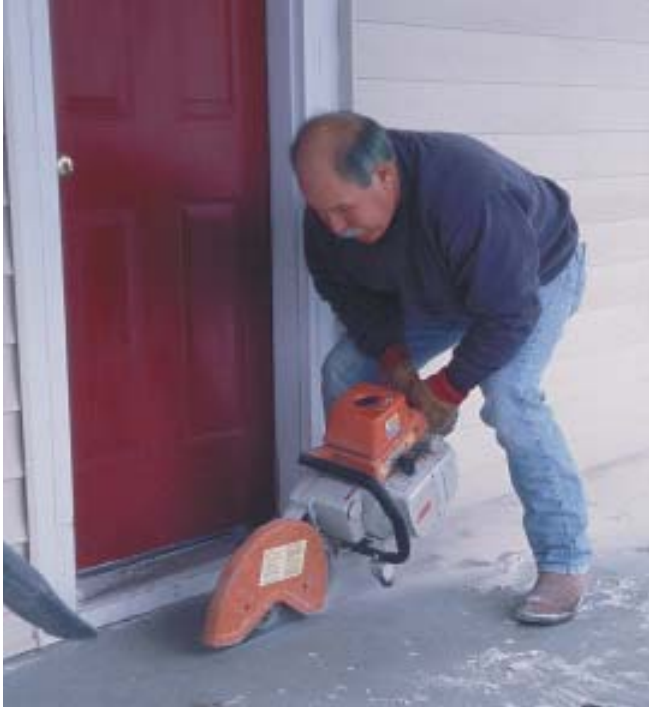
Figure 1. Cutting the existing porch slab prevented the concrete pieces from seesawing and damaging the siding. The crew used a leaf blower to remove dust and make it easier to see the blade and cut line.
