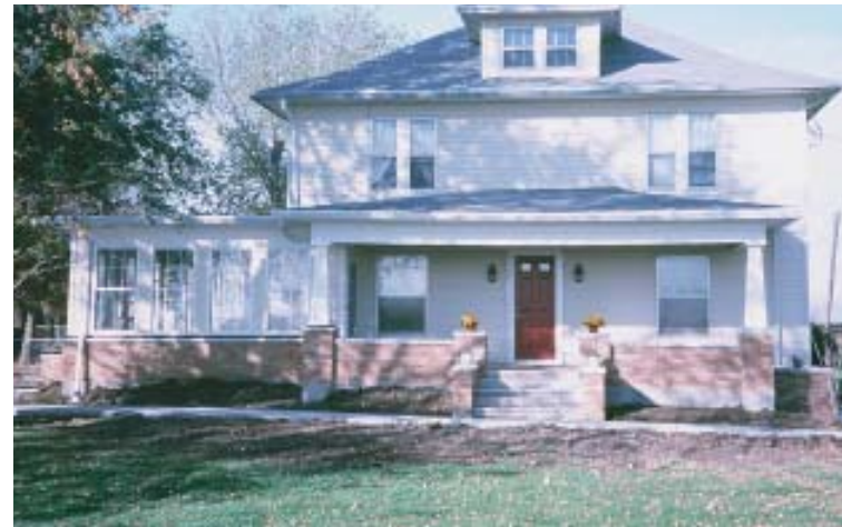
Figure 4. The heavily reinforced deadmen (top left) act as footings (top right) for the new front porch (above), which adds its weight to the resisting force.
