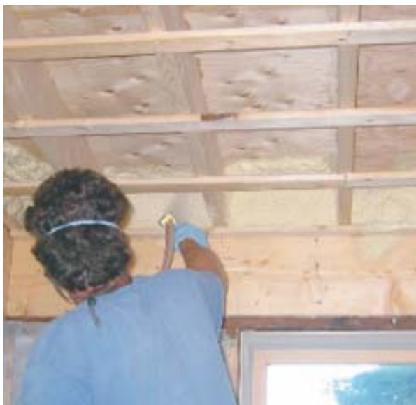
Figure 12. Two-component expanding foam seals and insulates in one step, making it an ideal solution for awkward configurations like this overhanging second-floor rim joist.
