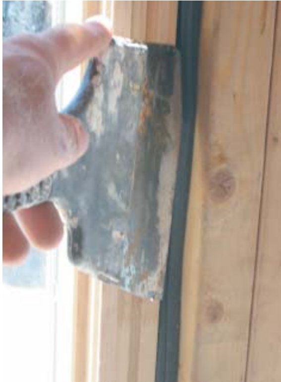
Figure 5. A compressible dual-tube rubber gasket, forced into the shim gap around windows and doors with a drywall knife, provides a highly effective air seal.
