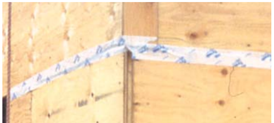
Figure 4. Instead of using housewrap, the author relies on plywood seam tape to block wind penetration. Tape installs easily just prior to siding.
