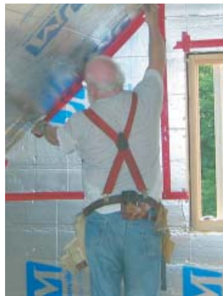
Figure 10. Foam board applied to the interior face of the exterior walls breaks thermal bridging through the studs and provides an effective air and vapor retarder.
