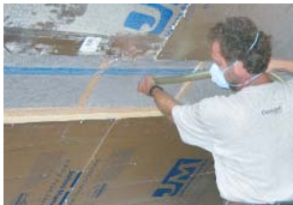
Figure 11. A narrow access strip in the middle of a cathedral ceiling insulated with rigid foam allows the author to view the bays as he fills them.
