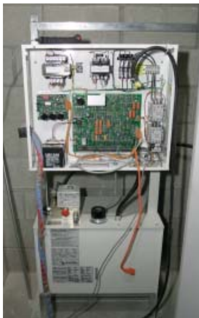
Figure 7. Sophisticated electronic controls tell the elevator when to start, where to stop, and how fast to go. The control panel in this machine room will be connected to a smaller panel in the cab.
