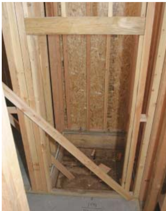
Figure 4. The bottom of the hoistway is dropped to accommodate the sling that supports the floor of the cab.
