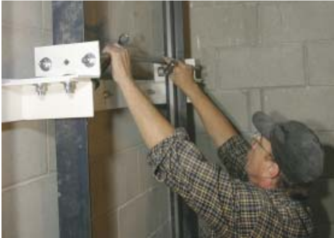
Figure 5. A pair of guide rails keep the cab aligned in the hoistway. The brackets that hold the rails to the wall can be adjusted in, out, left, or right. In the photo above, the installer is using a piece of conduit to gauge the spacing of the rails.
