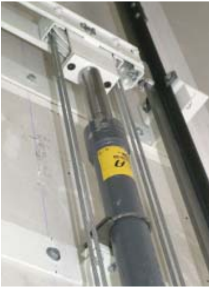
Figure 1. Roped hydraulic units use a piston to raise and lower a sheave. Cables pass through the sheave and connect to the sling that supports the cab. When the piston moves, the cab moves, too.
