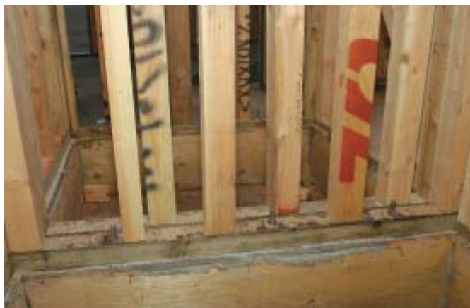
Figure 3. In a wood frame, one side of the shaft gets blocked for rails. Here the walls are blocked with vertical 4x4s, but some elevators require horizontal blocking, built-up members, or a hardware connection.
