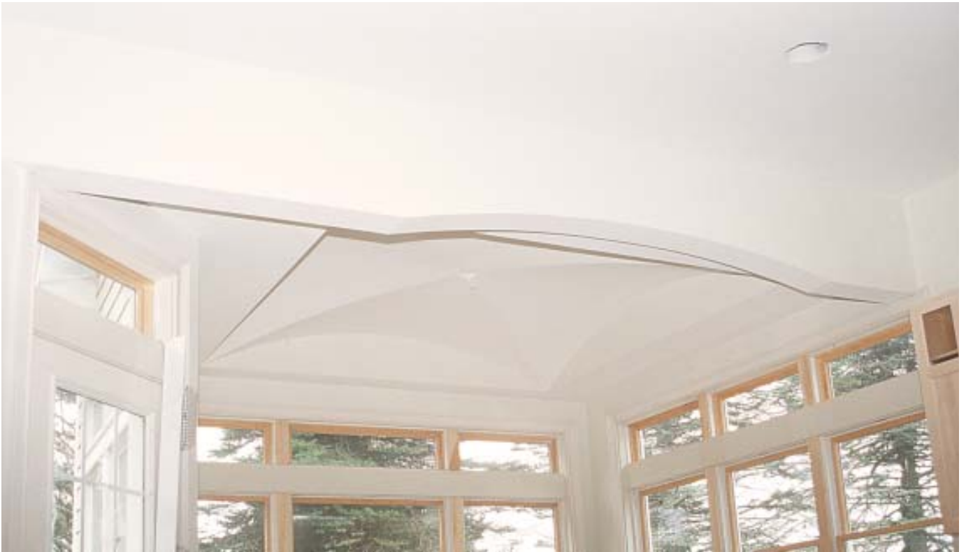
Figure 8. Thin \frac{3}{8} -inch drywall flexed without buckling over the concave barrel framing. To crisply highlight the lines of the cross-vault, the plastering contractor used expanded-metal plaster bead.
