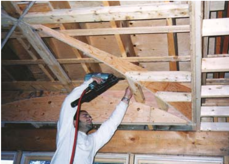
Figure 4. At the top of the groin, the ceiling blocks are square-cut at double 45-degree angles, but as the hip descends to the spring line, the cuts become progressively beveled. The author used a flexible story pole to space the blocking equally and divided the bevel angles incrementally between the top and bottom blocks.
