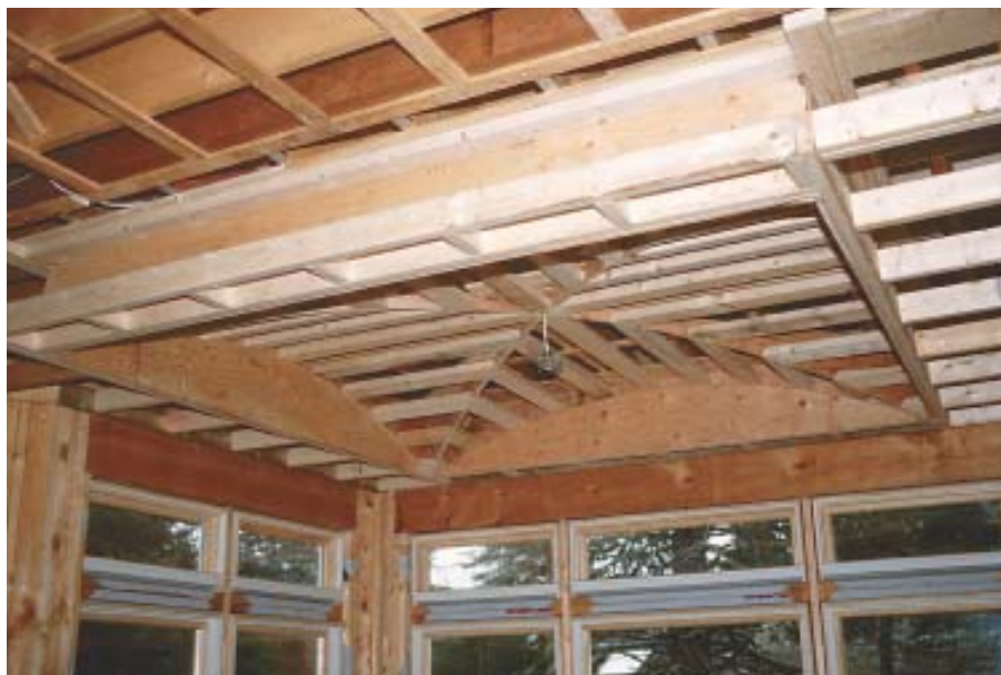
Figure 6. Although produced quickly, the vault framing is accurate, uniform, and almost too nice to cover up with drywall. The front soffit awaits a box-beam arch to complete the framing.
