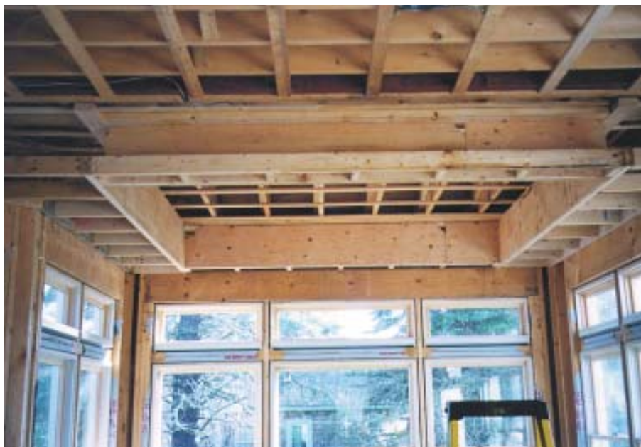
Figure 2. By dropping a perimeter soffit from the furred ceiling joists, the author created a visual division between living spaces and established a recess for the vault. Plywood backing on the vertical soffit faces provides solid nailing for the barrel arch construction.
