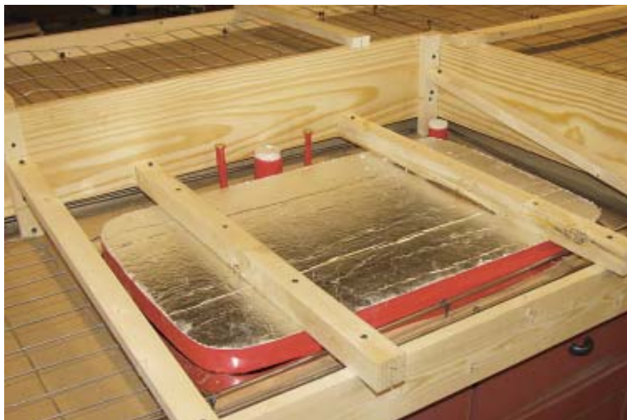
Figure 5. This foil-faced foam is blocking out the opening for an undermount sink. The foam and most of the wood forms pictured here will be removed as soon as the concrete is hard enough to finish. The undermount sink is already in place beneath the Kraft paper.
