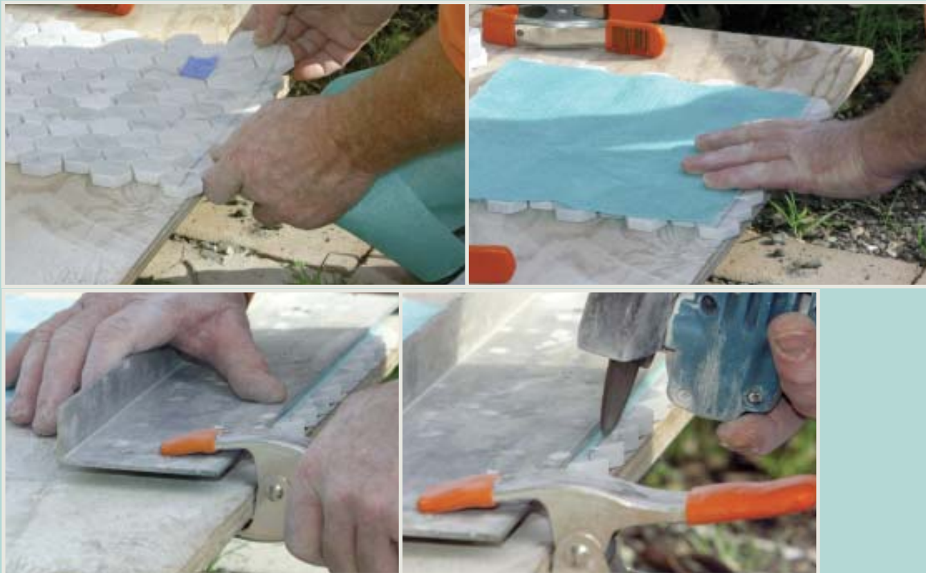
Figure 5. For cutting, the author clamps the small mosaic tiles to a workbench with an aluminum straightedge, using a thin piece of foam to protect the tile surface. He then dry-cuts to the line with a grinder.
