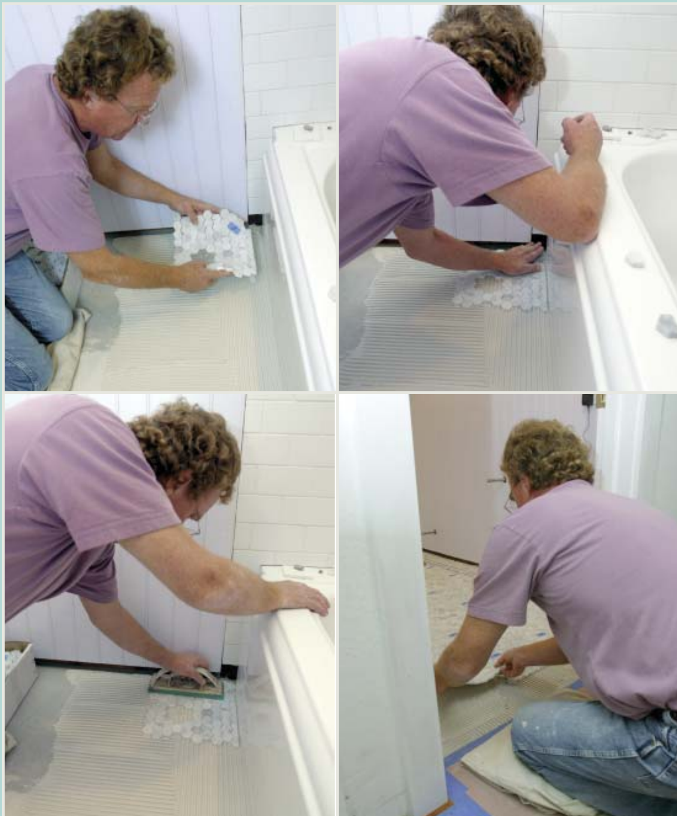
Figure 7. After placing the first mosaic sheet to a layout line marked on the tub, the author gently presses it into place by hand and with a rubber float. He takes care not to press excess thinset up into the grout lines, which would require time-consuming cleaning. Because the tiles were dry-fit first, the wet setting goes quickly.
