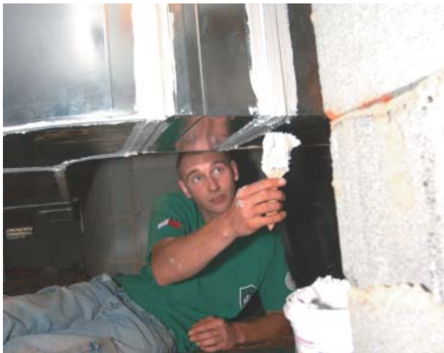
Figure 8. Thorough sealing of all duct joints is a critical quality-control step. Leaks in the ductwork allow moisture into the airstream, which will decrease system efficiency and may lead to condensation and mold growth inside the ducts. Applying sealant mastic with brushes or gloved hands is the preferred method for achieving airtight ductwork.
