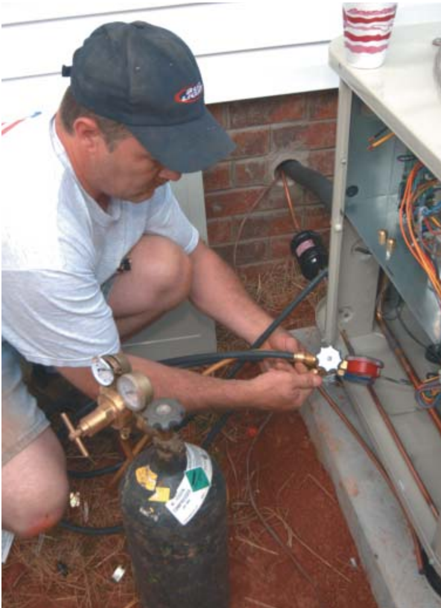
Figure 7. Before filling the system with refrigerant, the author purges the loops with nitrogen to eliminate moisture and oxygen that could corrode refrigerant lines and mechanical components.
