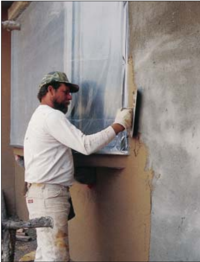
FIGURE 4. FINISH COAT. Code requires waiting at least seven days before applying a finish coat. Hairline cracks in this color coat are inevitable, but if the base coats are well cured, these surface cracks will not communicate water through the stucco.
