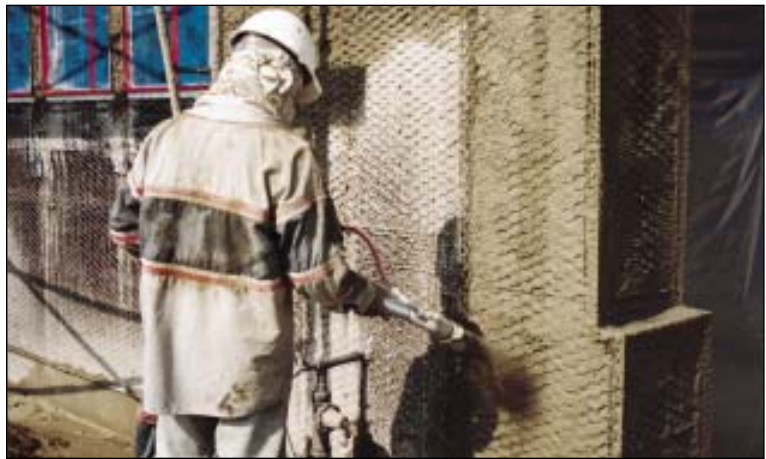
FIGURE 3. SCRATCH COAT. The first coat should be the hardest, using a rich mix. Stucco contractor Ron Webber recommends a Type II “plastic” cement without lime or other additives for the scratch coat. The mix will have no body and is hard to spread, but applying it with a pump makes this practical and results in the strongest possible base coat.
