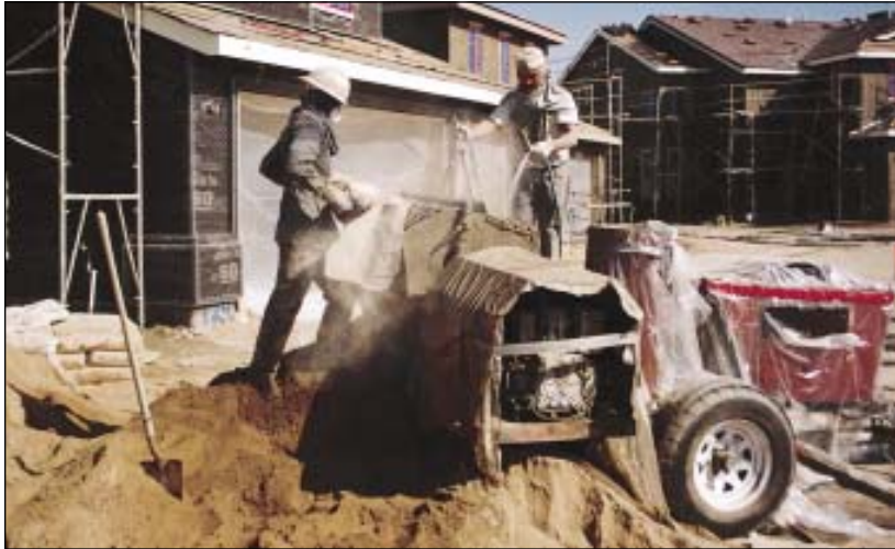
FIGURE 2. CLEAN SAND is as important to stucco as a low water-to-cement ratio and dry cement. “Dirty” sand, or sand intentionally mixed with clay to improve workability, will become porous as the clay dissolves, leaving behind air pockets. In humid climates, watch out for older bags of cement. Humidity can partially react with the cement even if the bags have never been opened.
