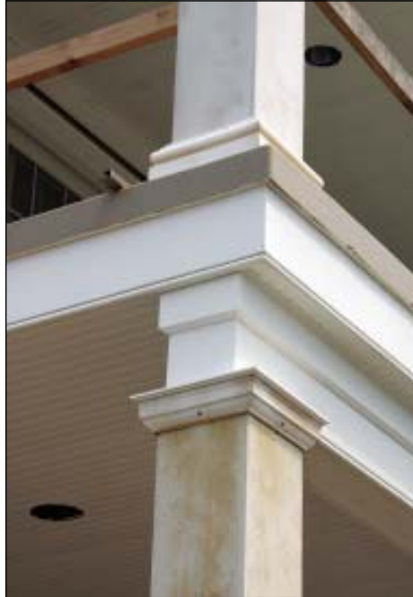
FIGURE 3. The porch's wood and steel structure is completely hidden once the porch receives its layered trim treatment of Azek ceiling beadboard, tooled Azek trim, and Fypon column base and capital moldings. In addition to its decorative purpose, the completed porch is able to shoulder its part of the design wind loads typical for a coastal home.
