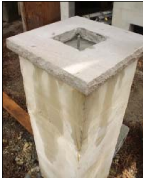
FIGURE 2. Column bases are tied to the foundation grid below grade. Above grade, Saduk's crews lay up 4-foot piers of 16-inch-square concrete masonry block, with fully grouted cores. Capping the block pier is a 20-inch-square bluestone slab, with a 6-inch-square hole in the center to receive the base of a 6x6 treated-wood post. The anchor bolt (top, center) will hold down a galvanized steel engineered standoff post base connector for securely attaching the wood post to the concrete pier. This block pier has already received a stucco scratch coat and will be given additional cementitious finish coats.
