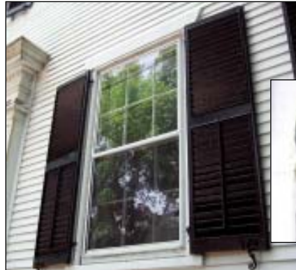
FIGURE 1. On the well-ordered facades of early American neoclassical buildings, exterior shutters play an important role in the overall design composition. Often called “blinds,” these exterior shutters hang on wrought-iron pintle hinges (inset) attached to the window frame.
