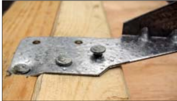
FIGURE 2. Nailers that drove the nail to the correct depth seated the nail as shown (photo center). When overdriven (photo left), the nail deformed the hardware, which is just as bad as under-driven nails (photo right). Deformed hardware and under-driven nails both result in an inferior structural connection that will not pass inspection.
