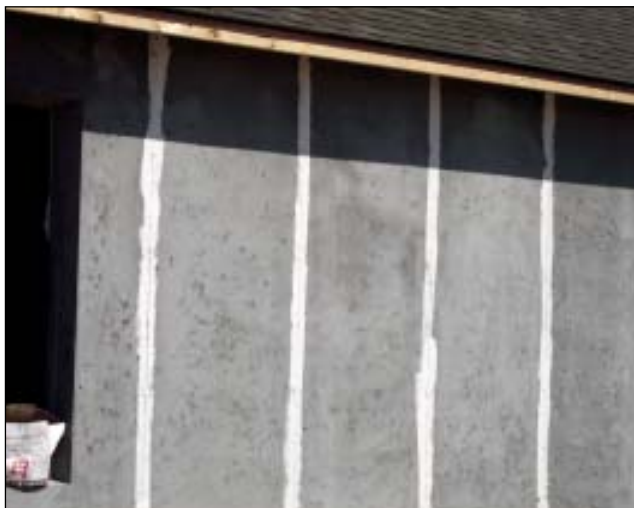
FIGURE 4. Form joints and snap ties are possible water entry points for wind-driven moisture. Applying sealant to these potential pathways is a simple, effective way to prevent water damage to the interior.
