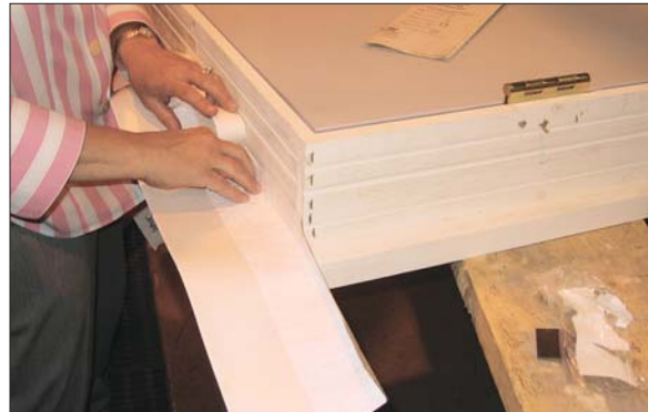
FIGURE 8. Tying a brick mold window or door unit into the drainage plane behind the brick presents a tricky problem. DuPont offers a flashing solution called StraightFlash VF — a peel-and-stick membrane that is applied to the back of the brick mold trim (top) before setting the unit into the hole (bottom). This way, brick mold casings can be integrated into building paper.
