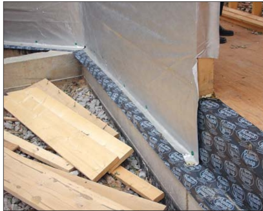
FIGURE 5. Good flashing is a key moisture management detail for brick veneer walls. At far left is a typical mistake: OSB sheathing layered over the top of a flashing membrane. Water seeping behind the brick will saturate and rot the sheathing. At left is a correct installation: the building paper has been shingled over the base flashing to direct water down and out.
