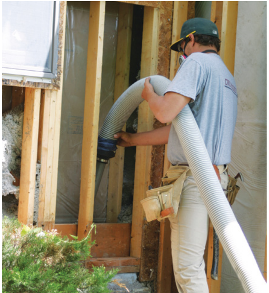
A Caleb Contracting crew member vacuums cellulose insulation out of a failed double-stud wall on a 1980s house in northern Vermont. Jim Bradley's crew is reconstructing the wall system after infrared and blower-door testing revealed major settling of the insulation, moisture damage, and pest infestation.
