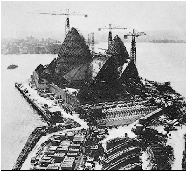
Construction of the "sails." Site precasting yards are seen in the foreground.
