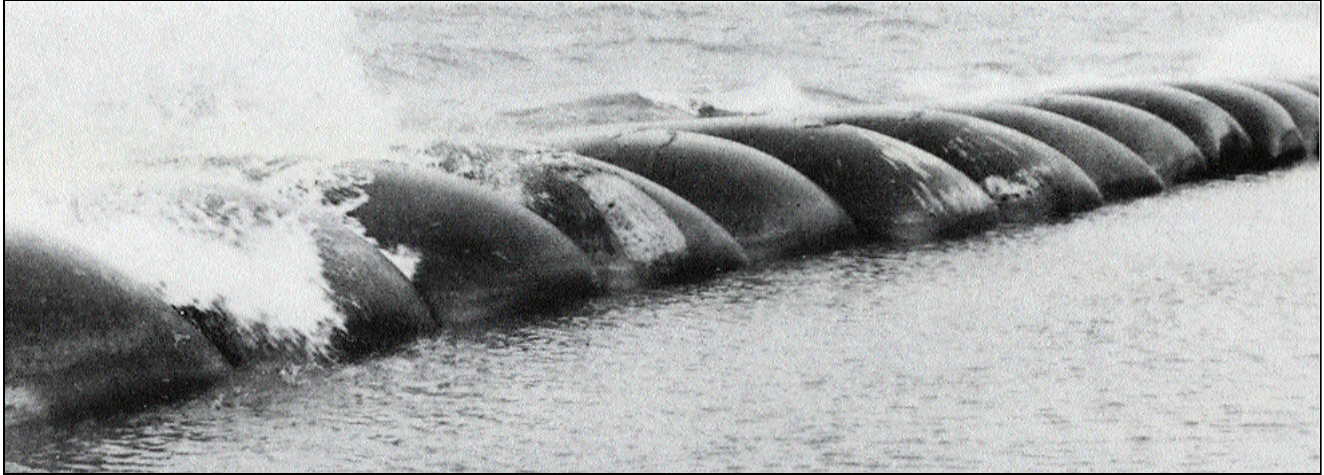
Shore protection made of blocks cast in place by pumping concrete into large fabric bags.
