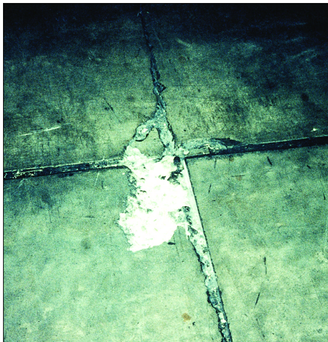
Joint fillers are too soft to support traffic across joints in industrial floors.
