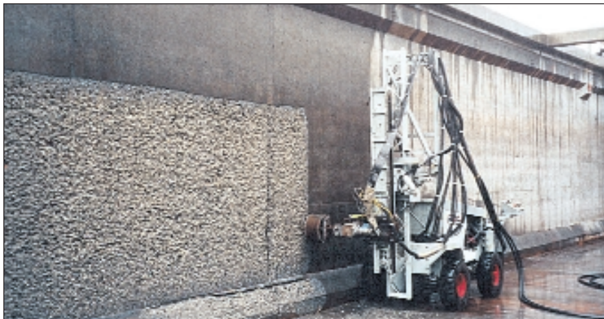
At the Secondary Waste Treatment Facility in Carson, Calif., a Programmable Logic Computer (PLC) was used to guide the nozzle to remove approximately \frac{1}{4} inch of concrete surface destroyed by acid from the sewage bacteria. A microsilica mortar was used to reconstruct the surface.
