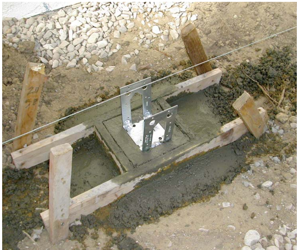
Figure 2. A string aligns the placement of a post base in wet concrete. Once the concrete has set, it will be easy to remove the form.
