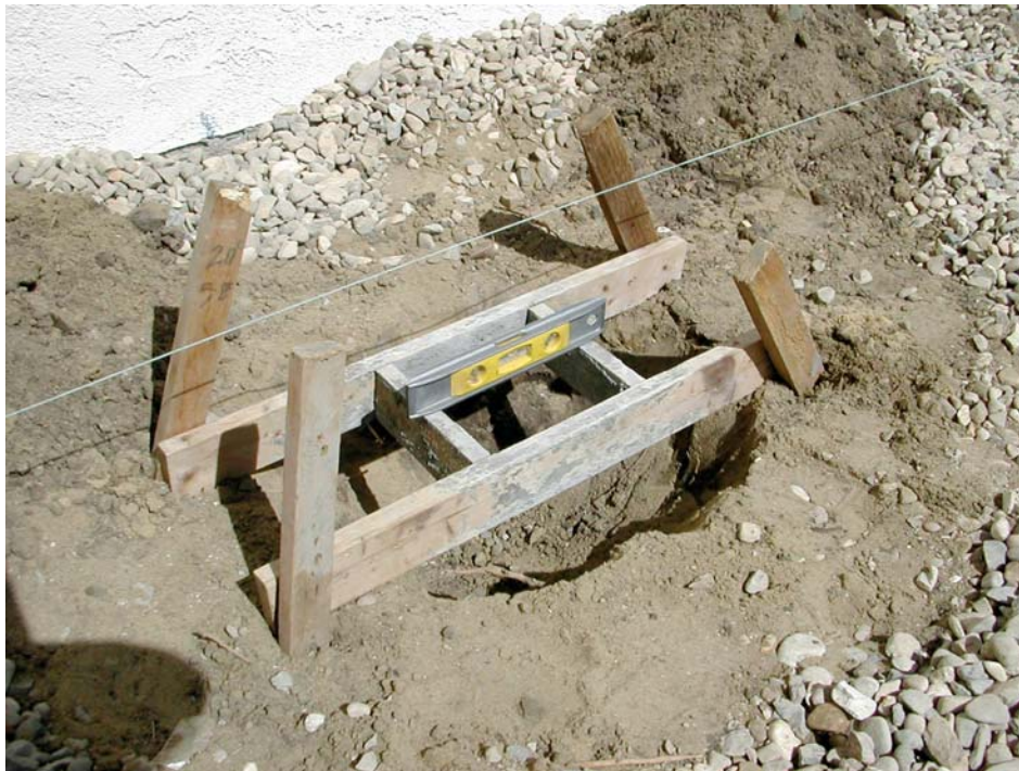
Figure 1. The form for the top of the footing is made from 1x4s fastened together at a slight angle. Four stakes support it and keep it level above the footing hole.
