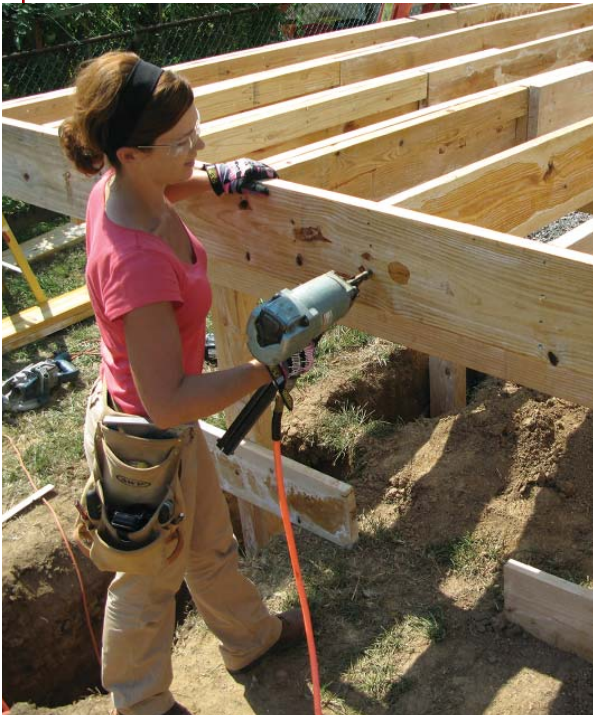
Figure 2. New this year, employers are required to provide personal protective equipment to their employees. This carpenter is dressed fairly typically for a job site, with safety glasses, gloves, and steel-toed boots. Yet she is only partway there — she's missing hearing protection and a hard hat. If she were working at a height, she also would be subject to fall-protection requirements.
