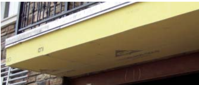
Figure 3. Building a deck that meets the IWUIC's 1-hour fire-resistive construction requirement is a challenge. Wrapping the structure with a Type X gypsum sheathing is one approach; additional cladding will be needed to protect the gypsum board from the elements.
