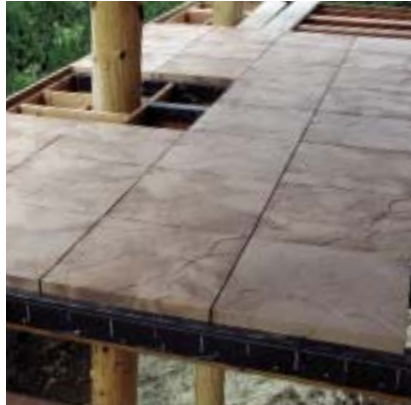
Figure 6. It's hard to figure out the code requirements for decking in the wildland-urban interface. For heavy-timber construction, the IBC prescribes a layer of T&G 3-inch-nominal decking topped by a layer of 1-inch-nominal T&G flooring run perpendicular – not a very practical application. Aluminum, tile (left), or precast concrete decking products, on the other hand, are inherently noncombustible.
