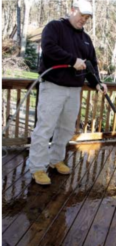
Figure 8. After the old finish has softened and lifted so it easily scrapes away (don't scrape caustic stripper with a fingernail!), a pressure washer sluices off the grunge.
