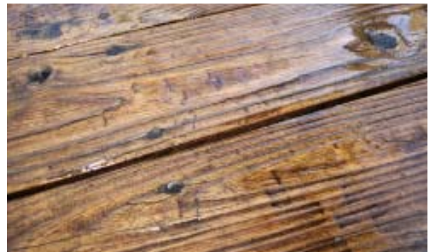
Figure 3. Be careful out there. The cross-grain scars on this decking were caused by a pressure washer being held too close to the wood.
