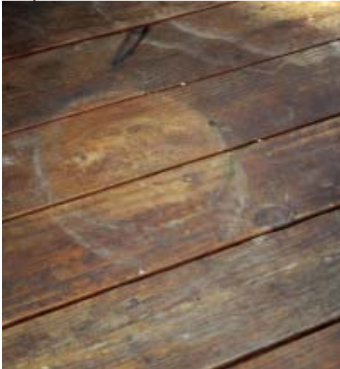
Figure 2. Cleaners make quick work of common finish problems such as stains and mildew. Items like potted plants, patio heaters, or grills leave stains. Mildew and fungi grow on damp wood, fed sometimes by linseed-oil-based finishes.
