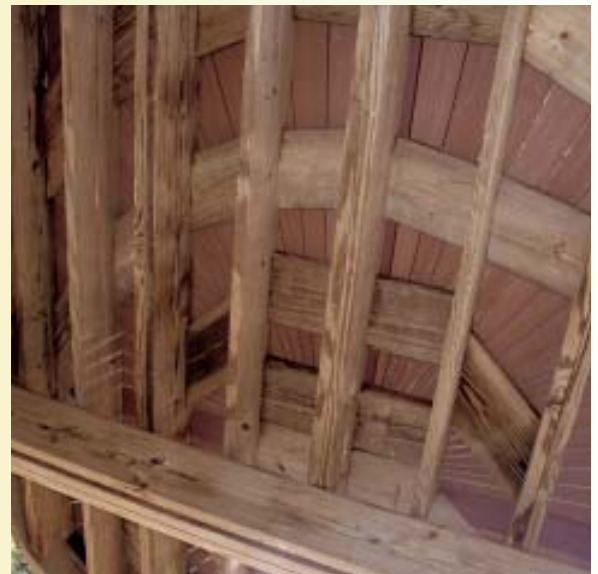
Figure 9. Some decking in the fan shape runs parallel to the joists, and the need for blocking to support it is obvious. Additional blocking allows the decking screws to be installed in concentric circles.
