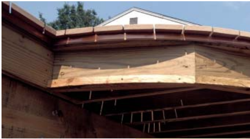
Figure 7. Notched to bend, an aluminum drip edge is installed below the decking to prevent streaking of the fascia. Bituminous roofing membrane on the joists prevents direct corrosive contact, and more membrane atop the drip edge seals the notches.
