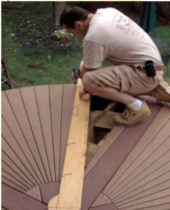
Figure 11. Another jig aligns the wedges radially. Cut to mirror the angle of the wedges, this second jig revolves on the center point.
