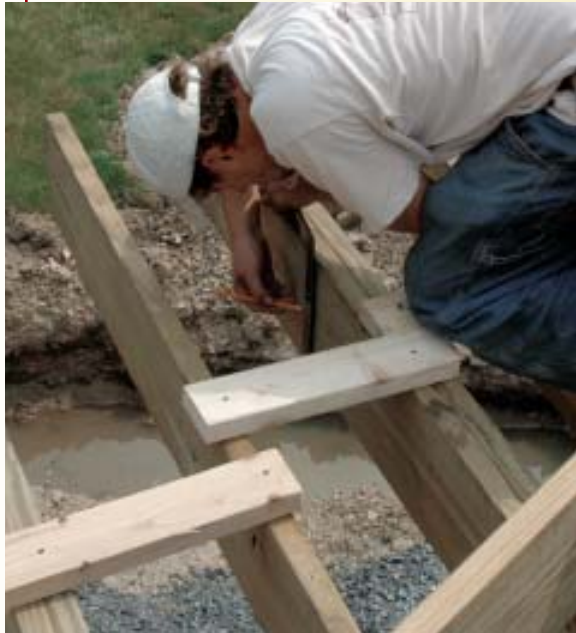
Figure 5. Mark the cut lines square down from the tops of the joists. The bevel angle for the saw is measured with a speed square from the marks atop the joists.
