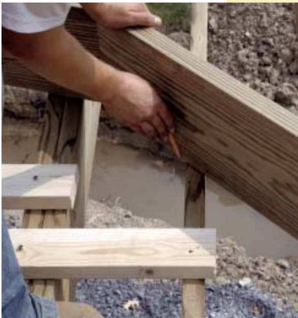
Figure 4. The cantilevered joists are purposely run long. The band board, aligned with the main deck, is placed atop the joists, which are then marked to be cut to length. Cleats nailed to the joists prevent them from moving and help to ensure accurate layout.
