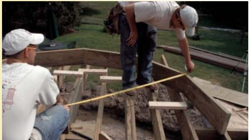
Figure 3. Always double-check the band board's size. The distance from the points of the miters to the center point of the curved section should be equal to the radius.
