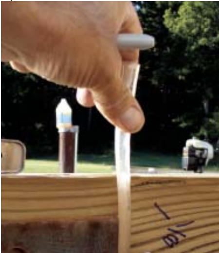
Figure 4. Marking directly from the fluid level is the most accurate approach to using a water level. However, you can also clamp the first end at a convenient height and measure up or down to the target level. Then, on the end whose level you're setting, just measure the same distance and mark.
