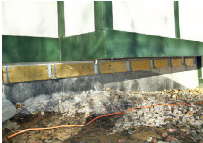
Figure 9. Attaching a deck ledger to the foundation has the added benefit of placing the ledger below any building cantilever.
