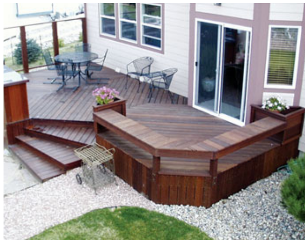
Figure 4. The surface of this bench seat is more than 30 inches above grade, but the deck surface isn't. Therefore, no guards are required for this deck design.
