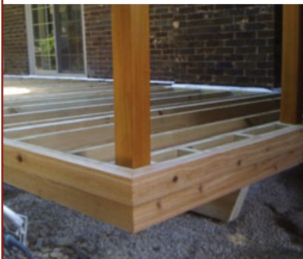
Value details can be simple, like this tiered fascia consisting of a 1x8 with a 1x4 cap.
