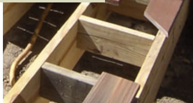
Figure 10. Where the border runs perpendicular to the joists, blocking is required for support.
