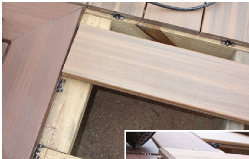
Figure 22. The ends of field boards fitting between two perpendicular picture-frame boards are fully slotted to slide into place over the hidden fasteners (above). Beveling the bottom of the field board allows it to clear the hidden fasteners' screws (right).
