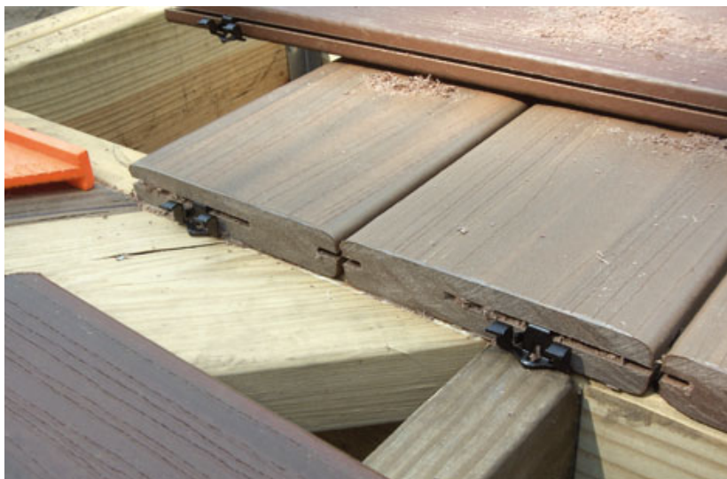
Figure 20. Slots cut in the ends of field boards accommodate the hidden fasteners for perpendicular picture-frame boards.
