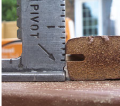
Figure 7. When deck boards aren't uniform, the precise fits required for a picture frame are more difficult.
