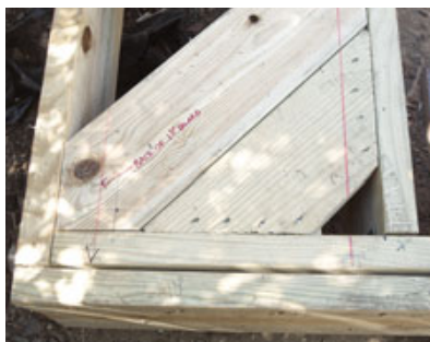
Figure 11. Corners often require solid blocking to fully support the ends of the deck boards.
