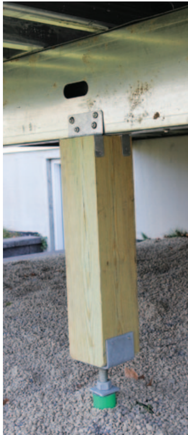
Figure 13. Wood support posts attach to LGS beams with hardware that's similar to what would be used with wood framing.
