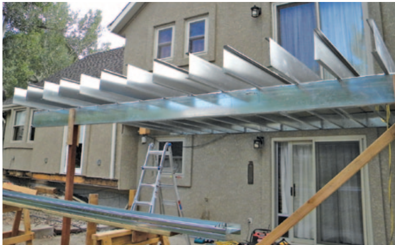
Figure 3. Although steel can span considerably longer distances than wood, it's only about one-third the weight.
