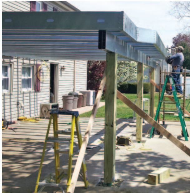
Figure 1. One big advantage steel framing has over wood is that its greater spans allow the use of fewer footings.
