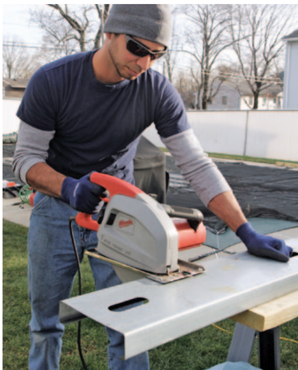
Figure 7. A specialized steel-cutting saw makes quicker work of cuts and does a better job containing the hot chips of steel from the cuts.
