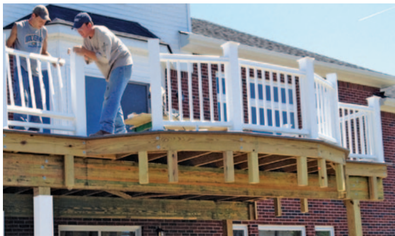
Figure 5. To support the fascia, blocking made from pairs of offcut 2x4s is installed approximately every 2 feet, and as needed to accommodate the shape of the deck. The longer leg of each 2x4 pair is fastened to the perimeter joist from behind so that the shorter leg aligns with the joist face.
