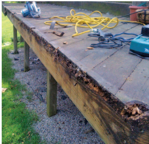
Figure 2. On this deck, debris trapped behind a flush fascia held moisture, which led to rot in the decking and trim.
