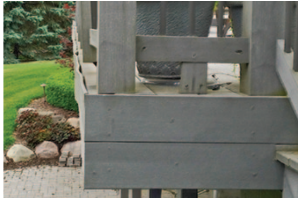
Figure 1. Water and debris that collect behind the fascia board can eventually cause it to pull away from the deck. Here the fascia has rippled and deformed at its top edge.
