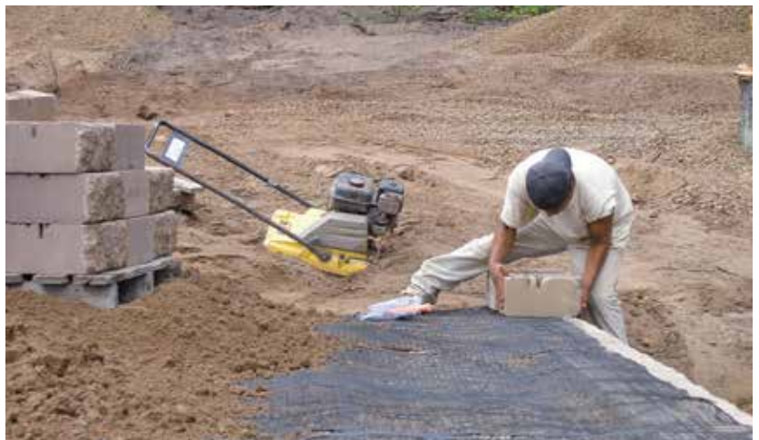
Figure 5. Synthetic geogrid is used when retaining walls are built on soils containing a lot of silt or clay, or when wall heights exceed four feet (top). The geogrid reinforces the soil mass behind the wall and helps anchor the block courses in place (above).
