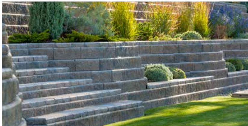
Figure 6. The first segmental retaining wall you build likely won't look like one of these projects, but the photos here illustrate the design possibilities offered by these versatile systems, including curved walls, planting areas, and coordinated paving-stone options.
