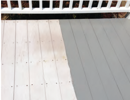
Prep work for a new Versacryl coating is similar to that for paint, with thorough cleaning followed by sanding.
