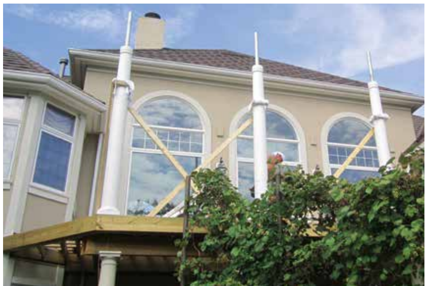
Figure 5. The lower columns were installed after the deck was framed (top). Workers added additional steel to the upper columns (middle) to provide a solid attachment point for the pergola and to resist both uplift and lateral movement (bottom). Each steel column has a steel plate welded to its base, which allows it to be bolted to the deck framing.
