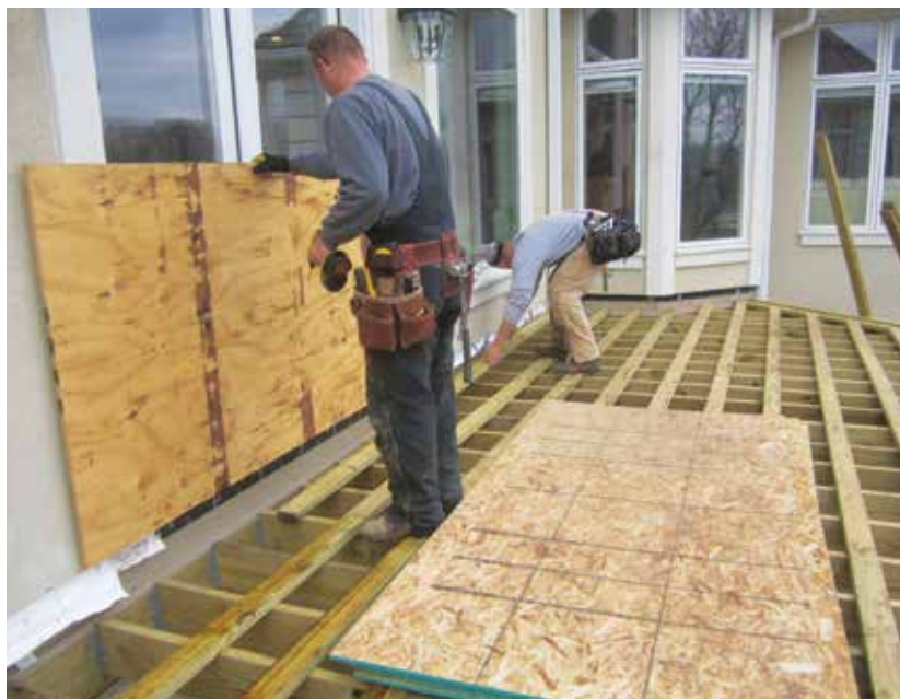
Figure 4. The new deck was framed with joists 12 inches on-center. To support the pavers, workers then screwed 2x4 sleepers to the tops of the joists, also 12 inches on-center.
