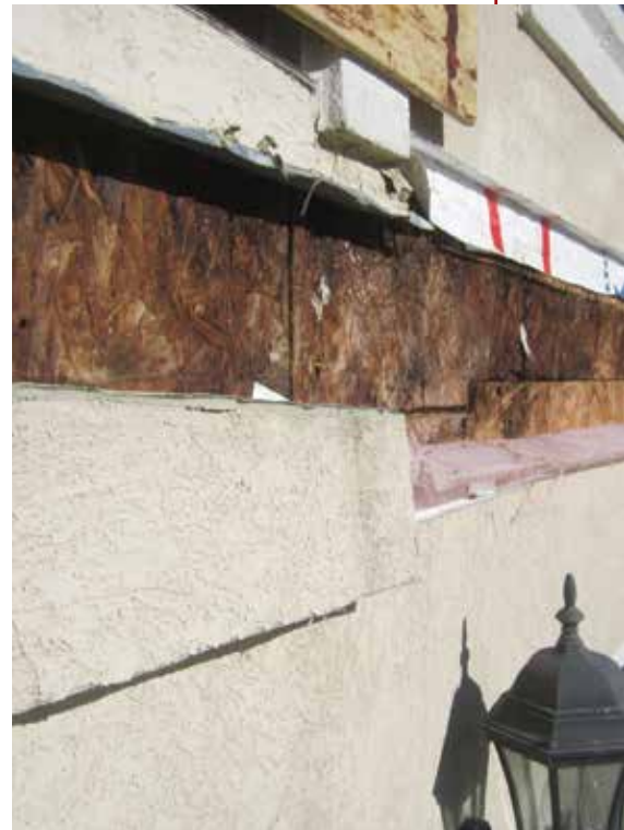
Figure 1. After removing the original cedar decking and framing (two photos, above), workers discovered moisture damage behind the home's EIFS cladding (right). The cladding had to be cut away to determine the extent of the damage to the sheathing and framing, and to make repairs.
