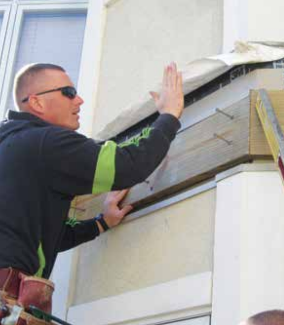
Figure 2. Before installing the new ledger, workers installed new metal flashing over the EIFS, and an SAF membrane over the sheathing.
