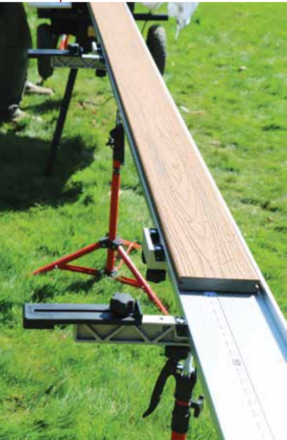
Figure 2. FastCap's optional molding stop is used here to keep the decking from sliding off the fence.
