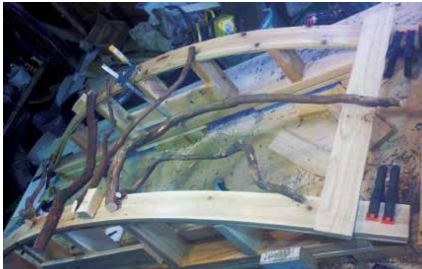
Figure 5. Assembly typically begins with longer branches left over from a previous section. Coped cuts are sometimes required where large branches intersect. To avoid splitting the branches, the author fastens them to the rails and to each other using galvanized 16-gauge finish nails.
