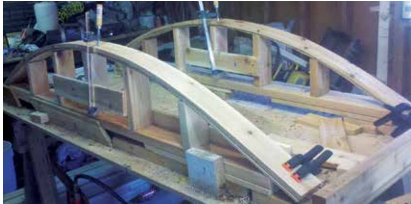
Figure 4. The building jigs are assembled out of 2-by lumber and 1/4-inch plywood. Here, curved top and bottom rails are clamped to the jigs.
