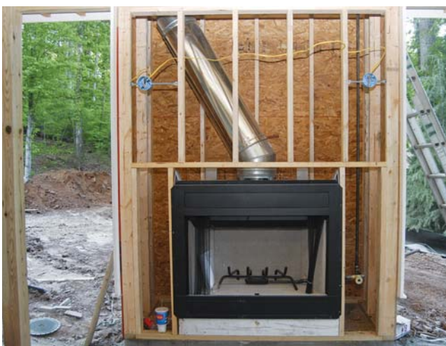
Figure 6. Stacked fireplaces begin with a ground-level masonry footing (above). The flue is offset and passes to one side of the upper fireplace (top).
