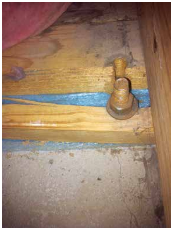
Inspect a sill plate carefully for structural issues before fastening a lateral load anchor to it.
