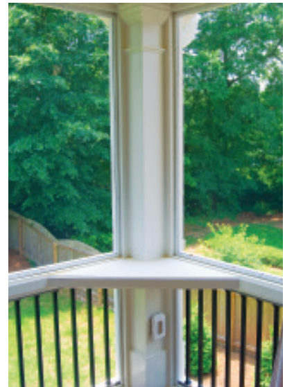
Figure 8. The beauty of PVC trim is its versatility; here it's used to create a maintenance-free corner nook on a porch.
